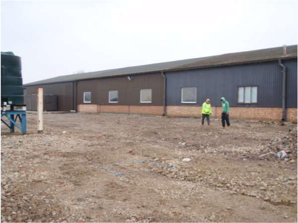
Plate 2. General view of site with post pads about to be excavated, facing north-east
