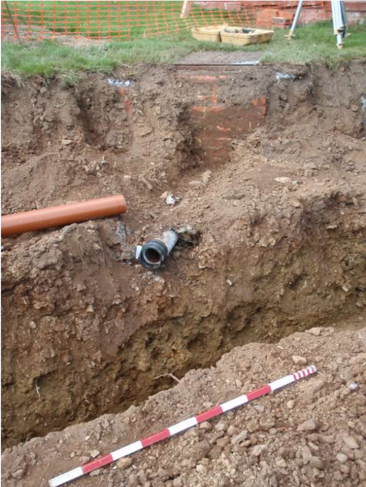
Plate 5. View of site showing service connections (looking south-west)
