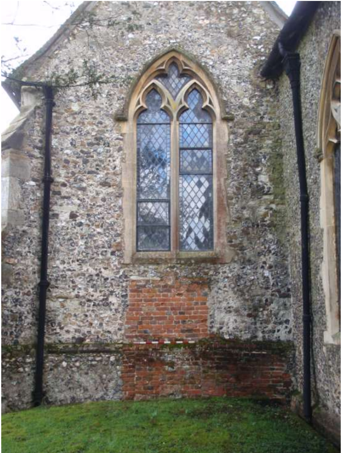
Plate 5. Proposed Development site showing blocked up doorway of proposed Doorway 1 (Looking east)
